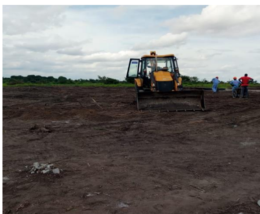
Figure 1: Initial civil works - cleaning the land to prepare construction of the Intermediary Medical Warehouse, Chimoio, Manica province.
