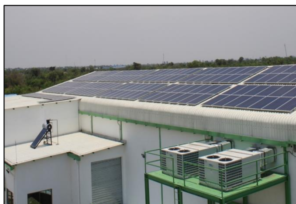
Fig. 3: Medical Warehouse Zâmbia, with Solar system installed. In Zâmbia, UNDP installed Solar Systems at all four Regional Hubs.
